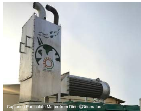
Capturing Particulate Matter from Diesel Generators
